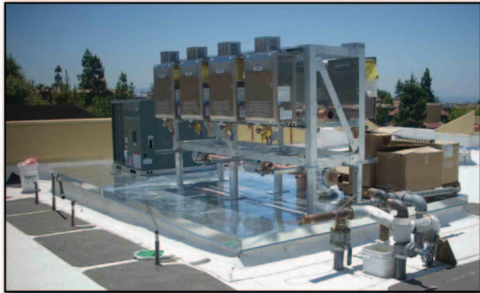
Designed by the P2S Engineering team, the racks were engineered to handle the required static loads and seismic forces. Adds project engineer James Valiensi of P2S: “Suttles Plumbing subsequently enhanced our design in the process of making it easier to build.”
